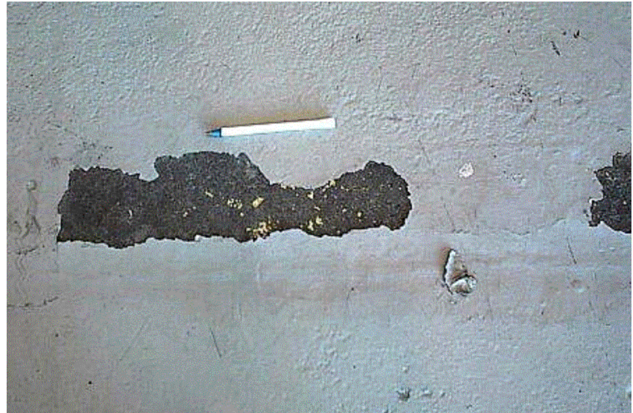
Paint chips and oil under coating
